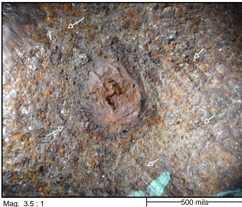
Figure 64: Failed location at 4 o'clock: An overall view of the corroded spot on OD. Arrows point to parallel line type surface impression around the corroded spot. Another view.
