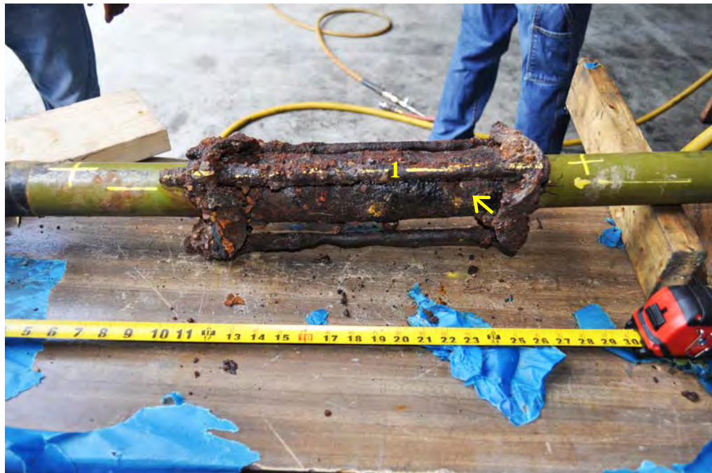
Figure 23: Arrow points to the 7 o'clock leak. Yellow lengthwise lines are witness lines. The cross-lines are cut lines.
