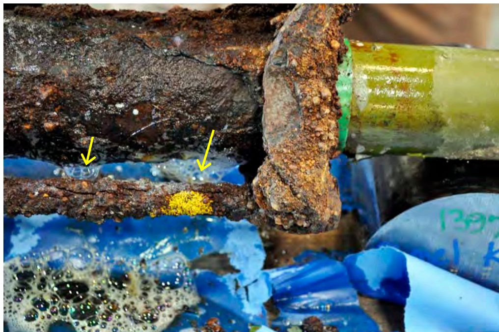
Figure 21: Another view of the leaking areas.
